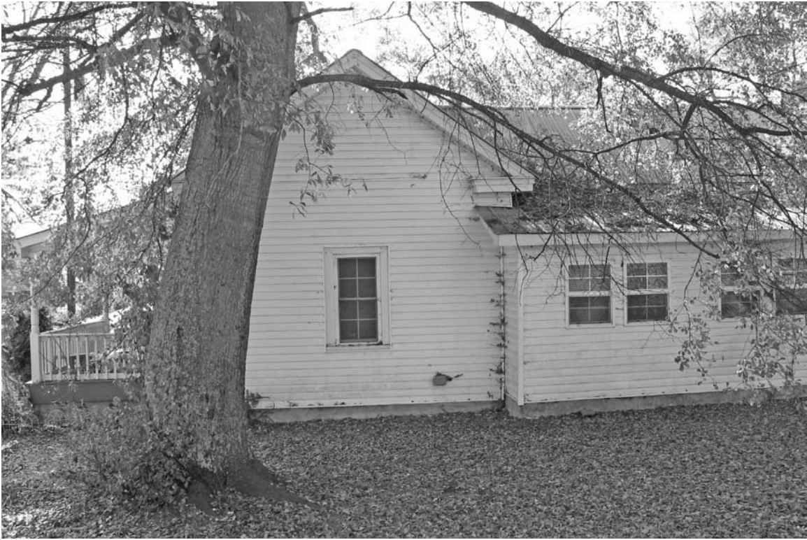
Photograph 3: View looking at the front portion of the right side elevation of the resource.
