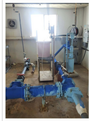
Inside of a Well House
